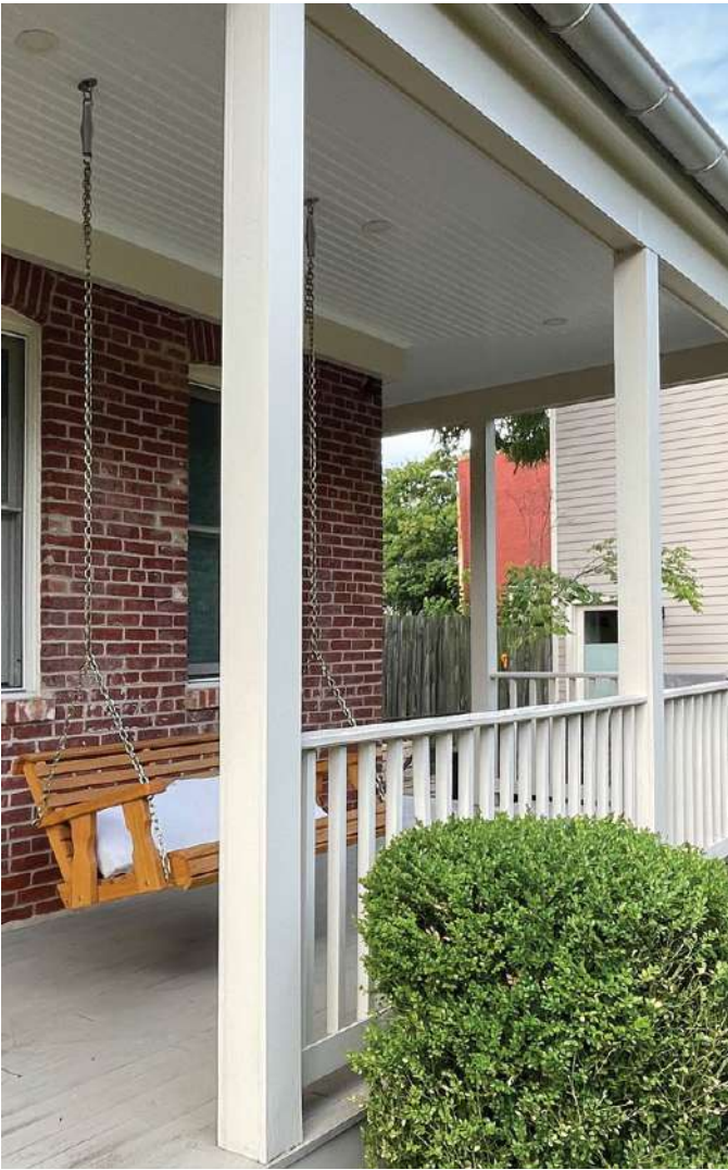
Figure 22. A porch was reconstructed using posts fabricated on site from a smooth-surface cellulose/polymer composite material. Though the face of the posts are painted, the lack of paint on the bottom at the cut ends is not consistent with manufacturers' recommendations. This treatment will allow moisture to be absorbed, shortening the life of the new replacement feature. Photo: John Sandor, NPS.
