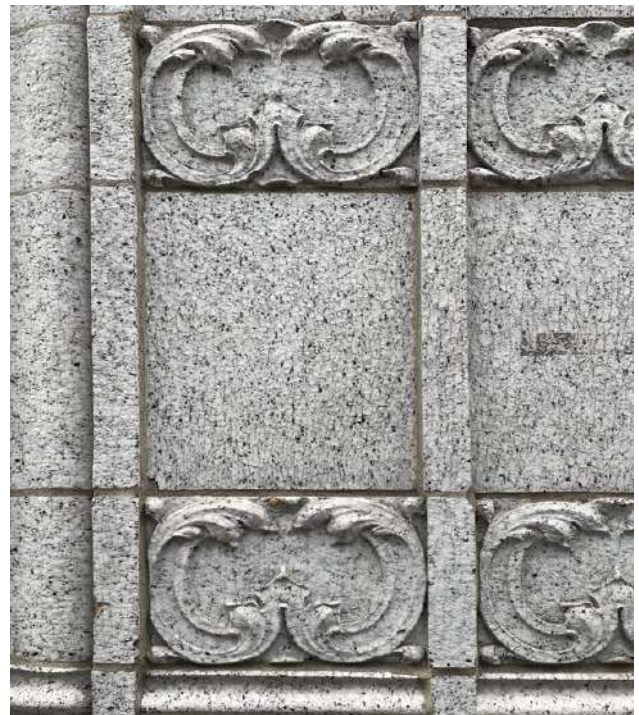
Figure 2d: Terra cotta gained popularity in the late 19th century as a cheap and lightweight alternative to stone. Glazing techniques allowed the blocks to imitate a variety of natural stone materials. Photo: John Sandor, NPS.
