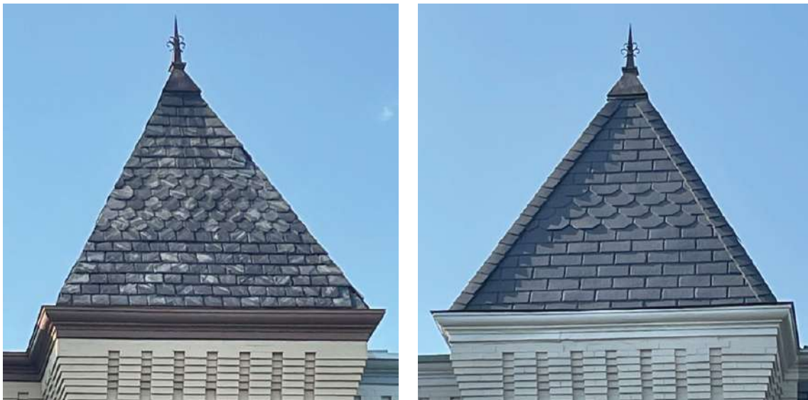
Figure 10. Polymer slates offer a choice of shapes but not sizes, limiting their ability to achieve a good visual match for some historic slate. With the size of the polymer slates (right) being nearly twice that of the historic slates (left), the scale of the entire feature is incompatibly altered. The molded edges of this material, which contribute to its ability to replicate slate, would be lost if each shingle was resized by cutting. Photo: John Sandor, NPS.
