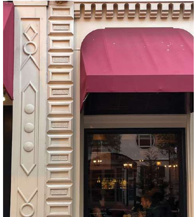
Figure 2b: The 19th century also produced a variety of metal products used to imitate other materials. Across the country, cast iron was used in storefronts to imitate stone. Photo: John Sandor, NPS.
